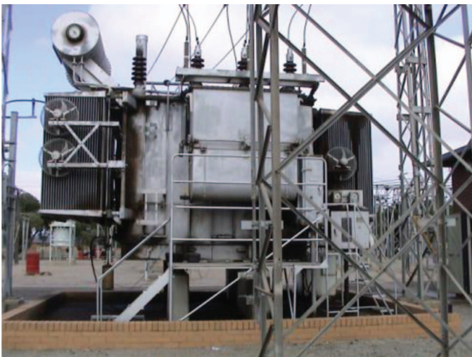
Figure 3. Transformer 1 used for this study.
